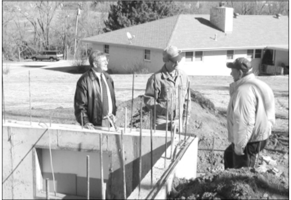
From left are Western Technology Center Assistant Superintendent Cliff Corbin, Cordell resident Roy Dewees, and Jerry Koehn, coordinator of the Cordell Skills to Rebuild program. Koehn is offering free construction training to Dewees and other Cordell residents who are rebuilding their homes after the October 2001 tornadoes.
