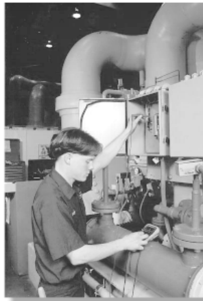
Paul Johnson, shown servicing an electrical panel at Oklahoma State University’s chill water plant, is a 1995 graduate of Duncan High School and the Red River Technology Center air conditioning program. Johnson is one of the youngest service technicians ever hired by Carrier Heating and Air Conditioning in Oklahoma City.
