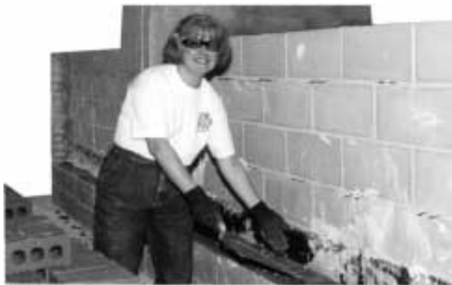
Danene Vincent, director of Instructional and Curriculum Services at Metro Tech, is pictured laying a brick wall during a Skills to Rebuild Class at Metro Tech's Skills Tech facility in Oklahoma City.
